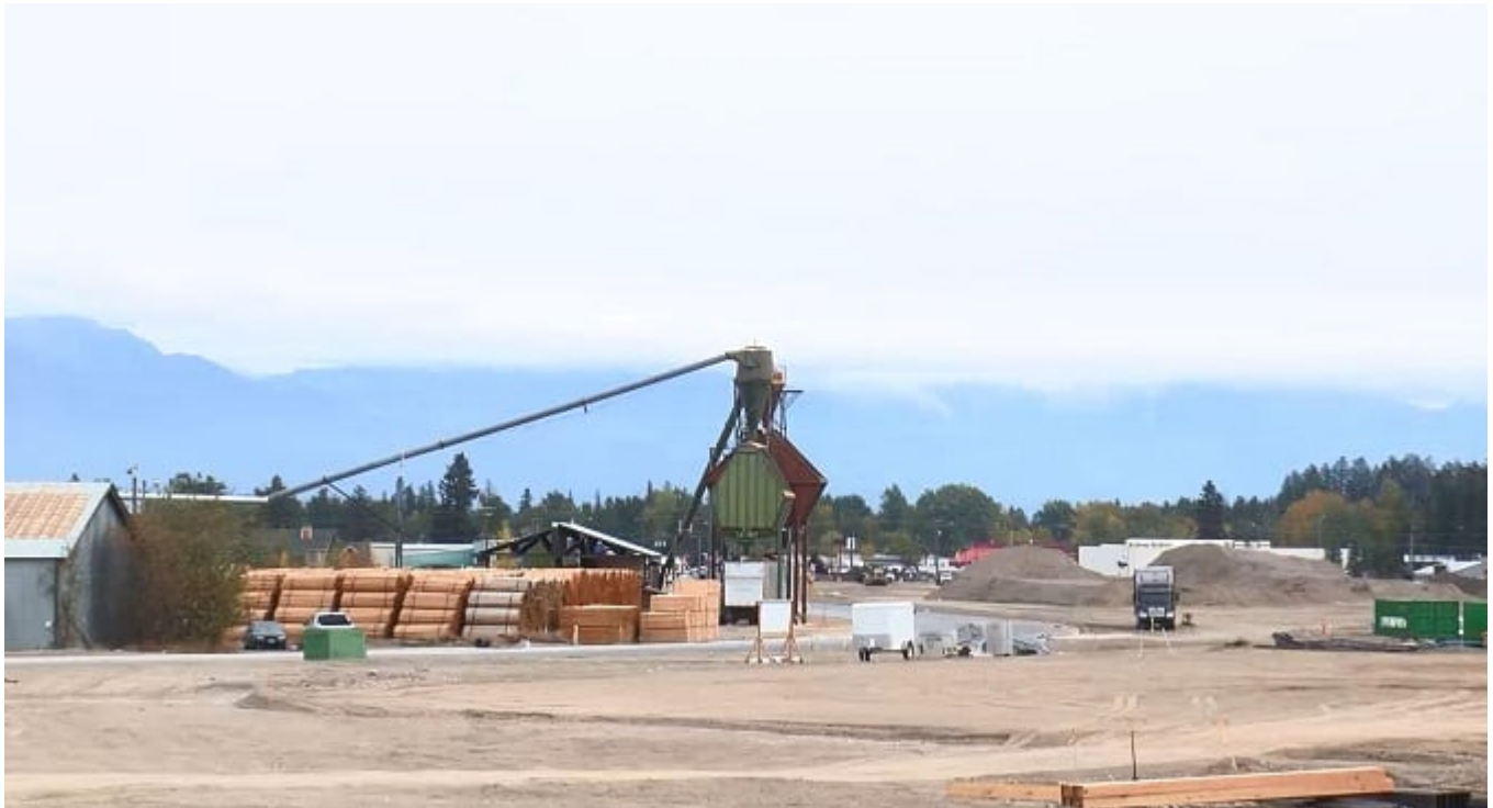
The site of the new Glacier Rail Park in Kalispell. (MTN News photo)
