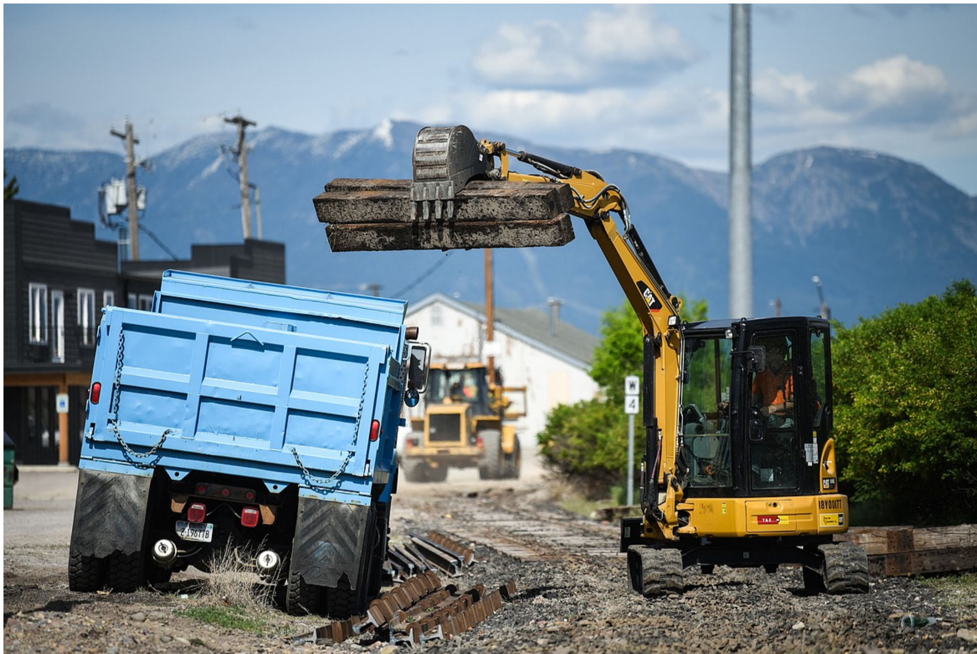
Crews remove railroad ties and sections of track near Fifth Avenue West North to make room for the Kalispell Parkline Trail on Tuesday, June 1. (Casey Kreider/Daily Inter Lake)
